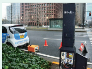
Supplying power to traffic lights (control panel shown at bottom right)
